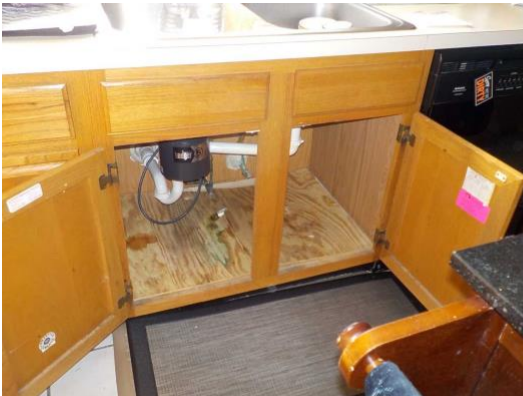
12-kitchen sink cabinet dmg
