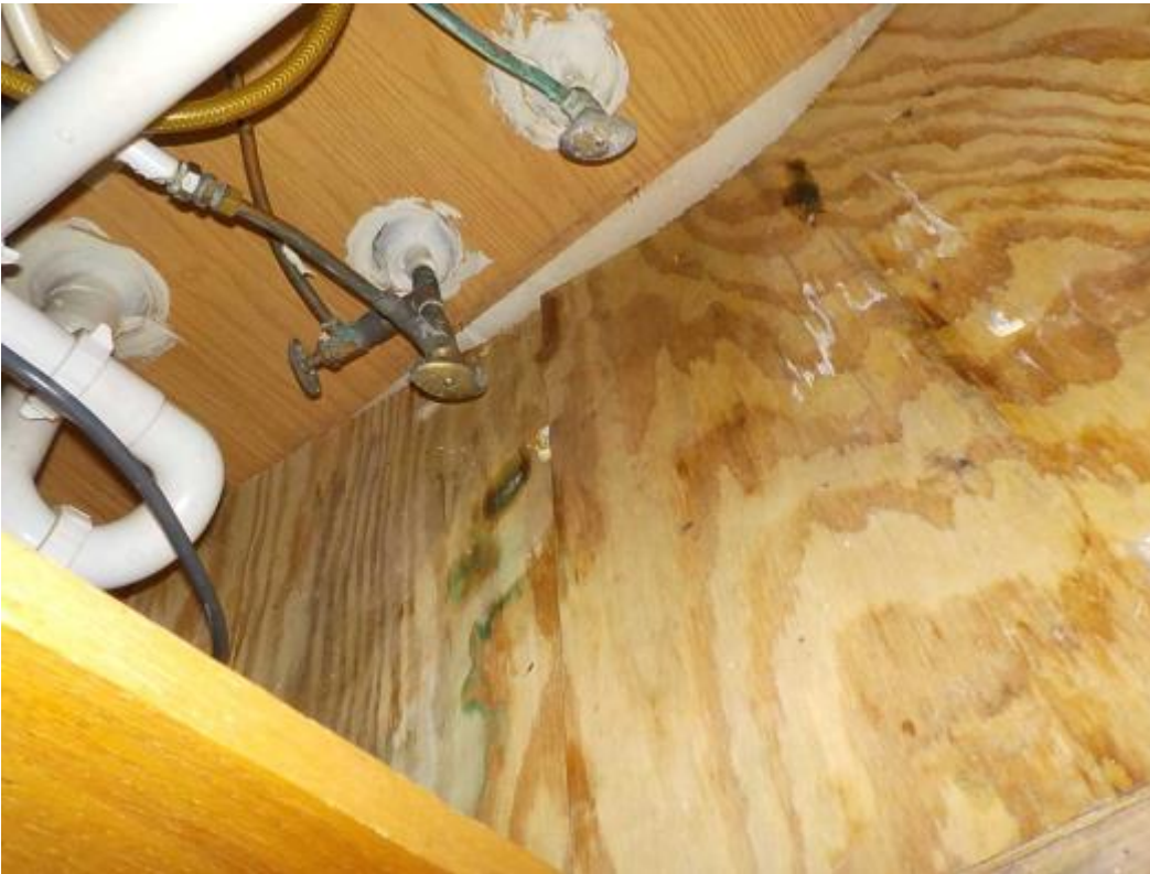
17-kitchen base cabinet damage
