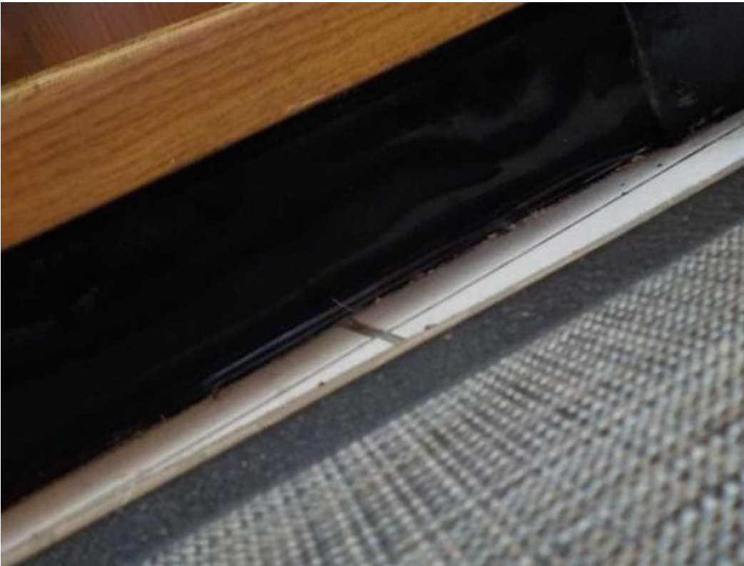
13-cove base on toe kick
