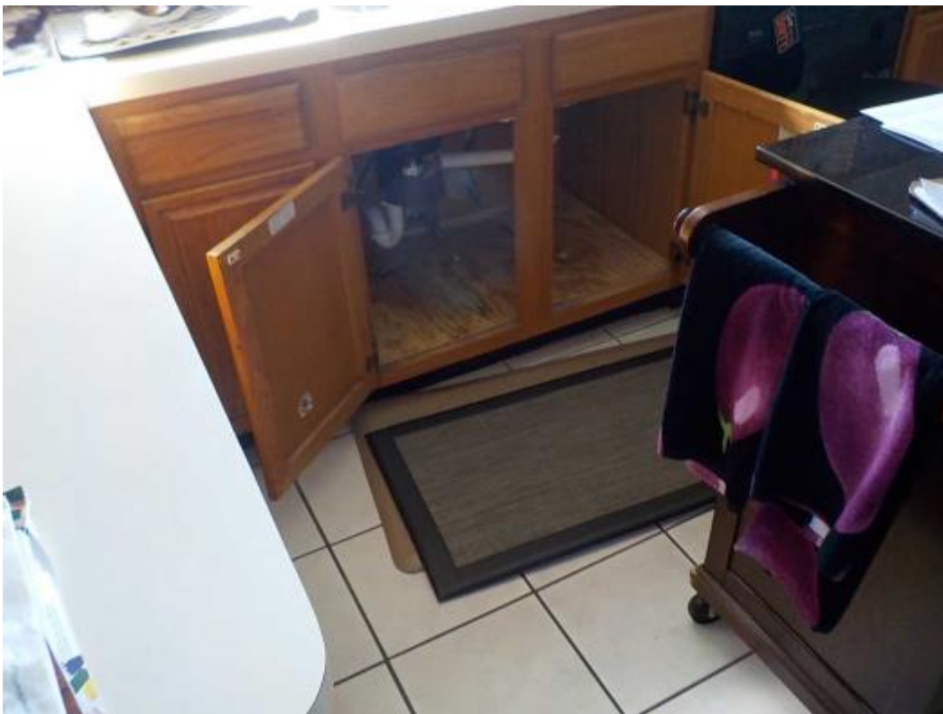
24-kitchen damage overview
